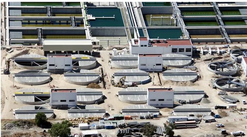
← Sludge Thickener Tanks
